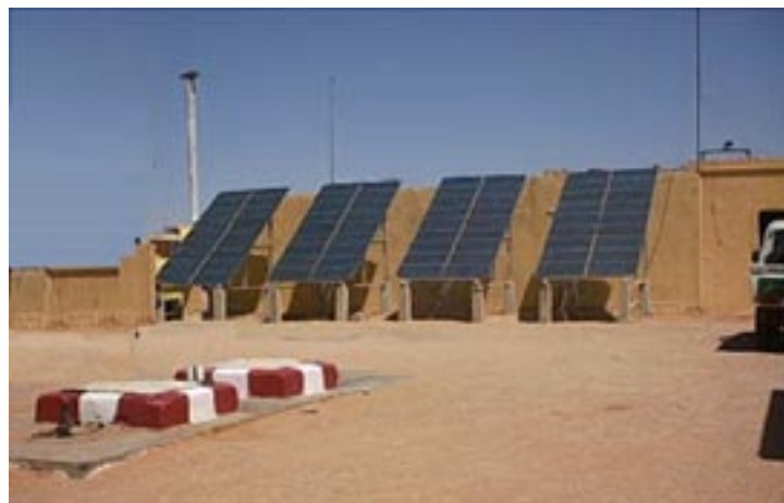
Le Champ Photovoltaïque
