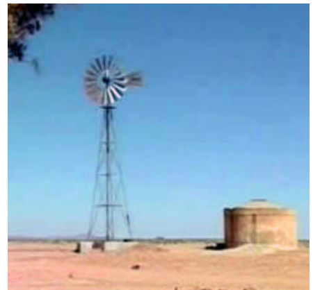
pompage éolien à had sahari Willaya de djelfa
