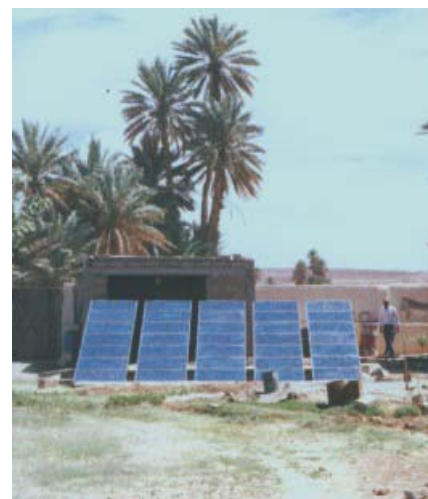
Installation de pompage photovoltaïque - Fendi W. Bechar
