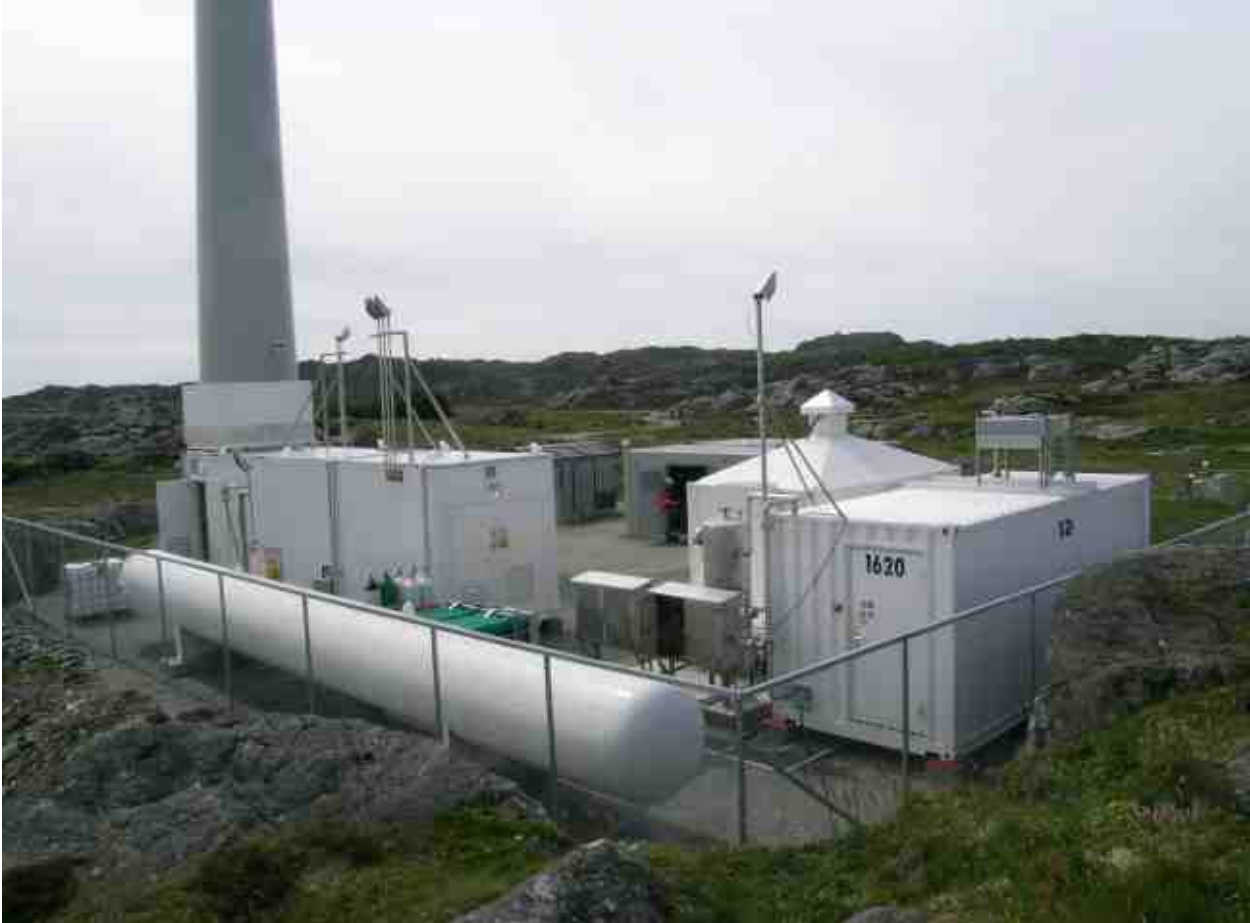
Figure 2: Photograph of the wind-hydrogen power plant at Utsira. To the left: the wind turbine tower. Below the tower: the electrolyser and compressor container. In the front: the H 2 -storage tank. To the right: the fuel cell and H 2 -ICE container. In the background: the grid stabilizing equipment.
